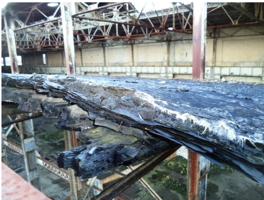
Photo #4: Typical Roof Deterioration
