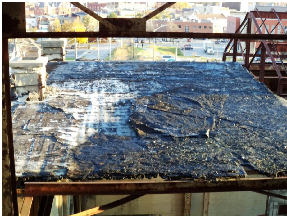
Photo #6: Typical Roof Deterioration
