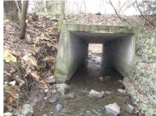
Scour at NE Corner
