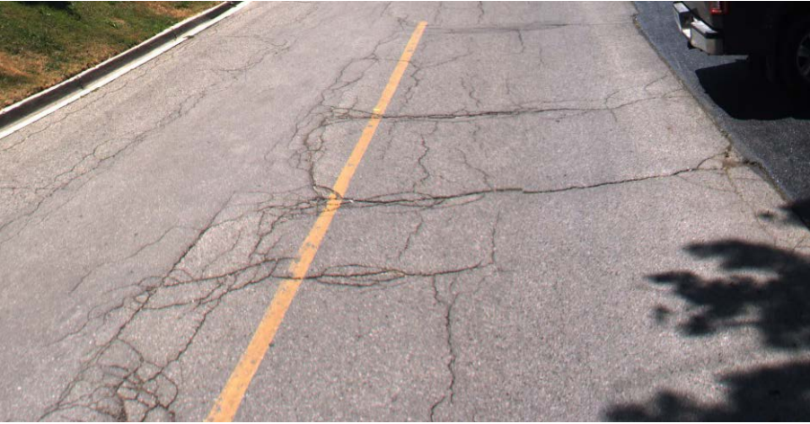
Cobourg St - Poor Road Condition
