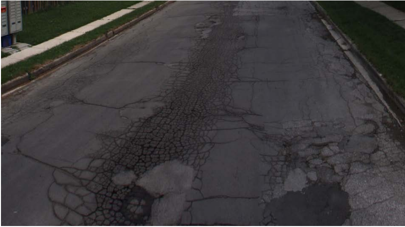
Player St - Very Poor Road Condition
